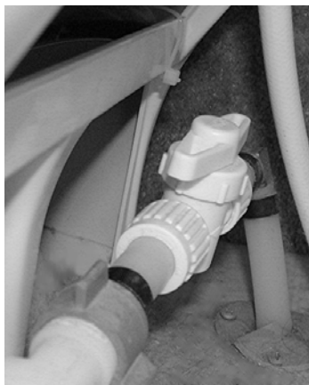
Photo 1: Shut-off valve on toilet
