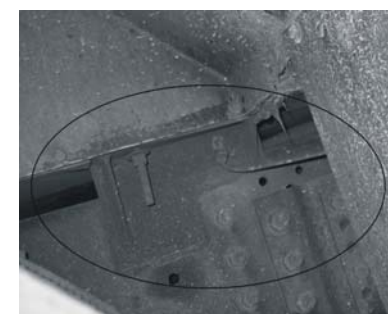
Photo 4: Passenger side bracket forward of the axle is cracked and the bolt is bent.
