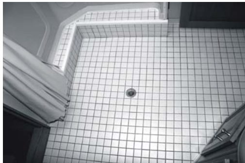
View of shower floor with realigned drain. Door to living area on lower left; to bedroom upper right.
